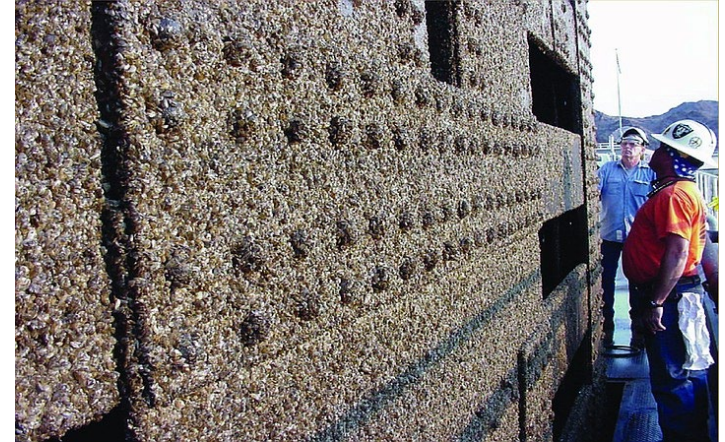
Invasive mussels fouling a penstock gate at Davis Dam. 📷 : U.S. Bureau of Reclamation
